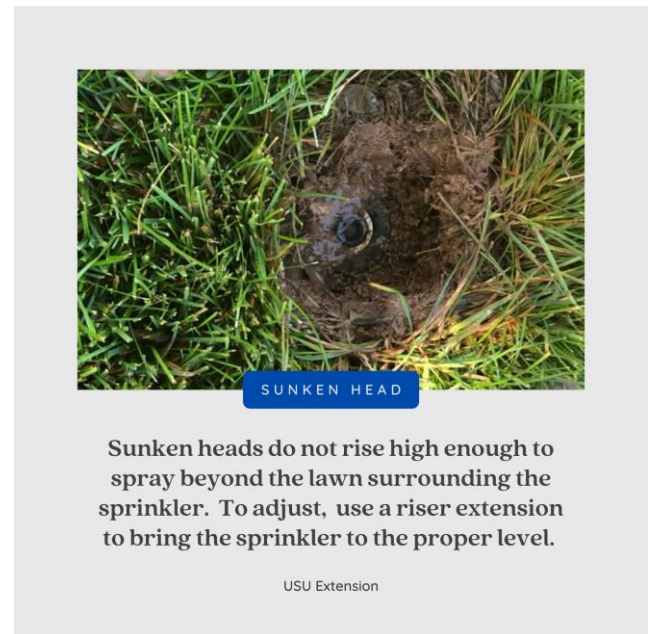
Figure 3. Sunken sprinkler head
