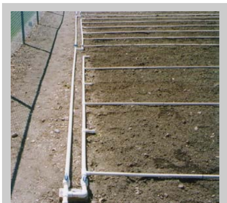
Main distribution lines are glued, lateral lines are not glued
