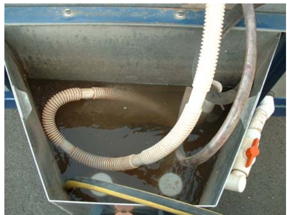
Picture F: Pump Compartment
