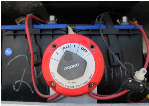
Picture I: Battery Switch
