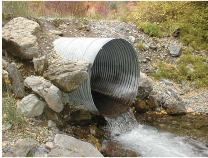
Waterfalls from culverts scour the stream bed and make fish passage difficult. Aligning the culvert with the stream gradient is the preferred practice, although rock armoring can be used here below the waterfall to reduce scouring and above the culvert to reduce road erosion.
